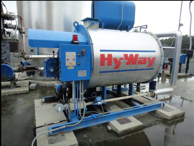
HOT OIL HEATER
